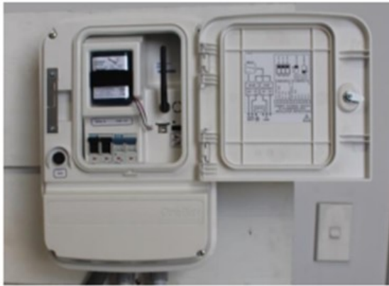
Figure 7: Example control panel
