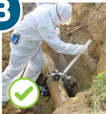
Chain pipe cracker
